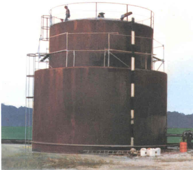
Storage tank with completely rusted surface.
