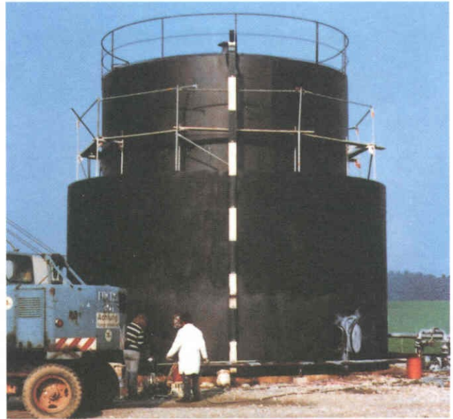
The same storage tank after applying noverox®: the rust was transformed into a black protective layer.
